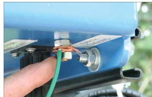
Close-up of earth ground lug.
